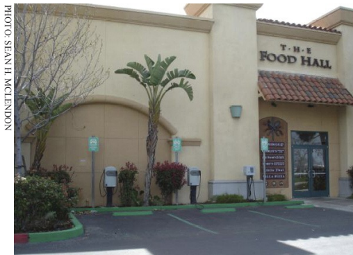
Electric vehicle charging station at the Camarillo Outlet Center in California is a prototype for the development of a recharging infrastructure.
